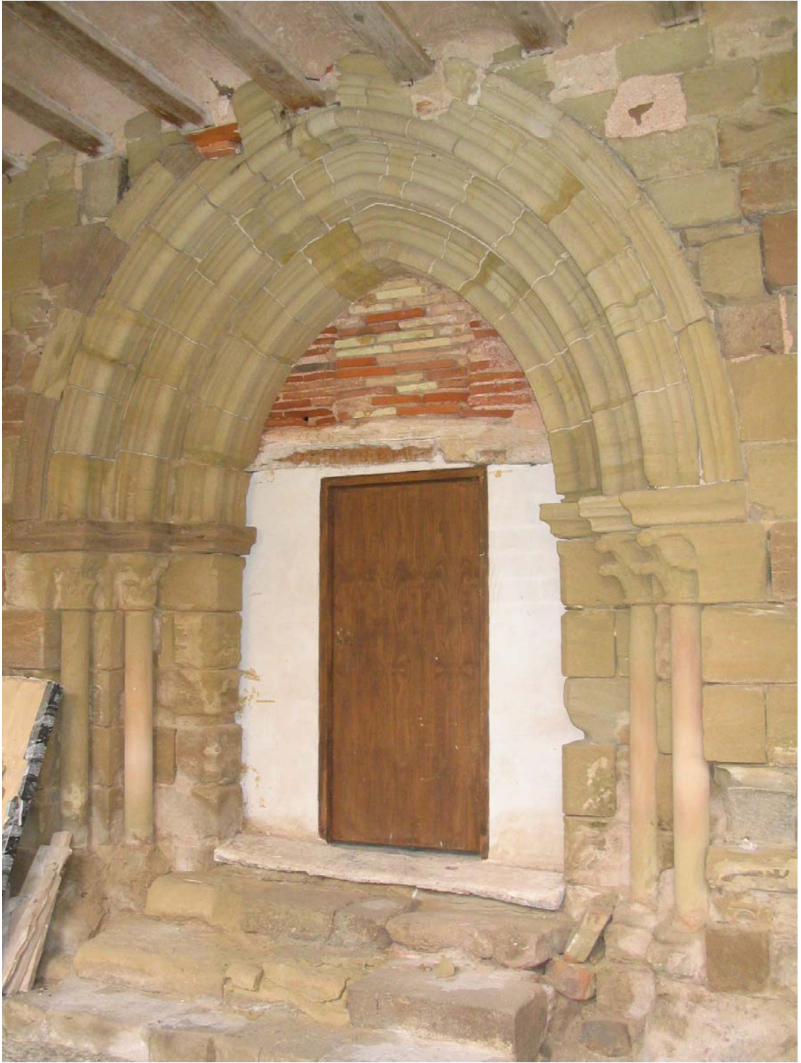
Fig. 26. Former entrance to Refectory and Kitchen from Cloister, Santa María de Cañas, c. 13 th century.
